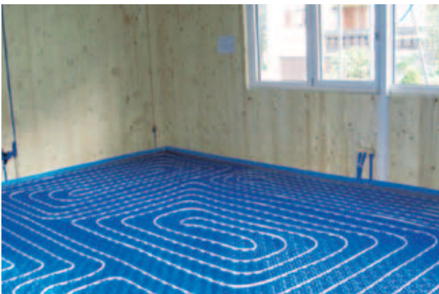
Fig. 15: Piping of an underfloor heating [with the kind support of Eberle • d e n k f a b r i k • Dornbirn, Austria].
