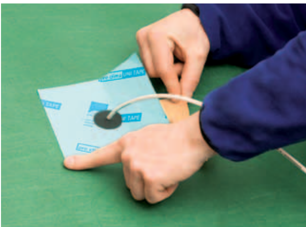
Fig. 10: If the penetrations cannot be avoided, suitable and approved systems should be used for sealing. A quick and permanently tight mounting will justify the additional costs [with the kind support of the company pro clima 2011].
