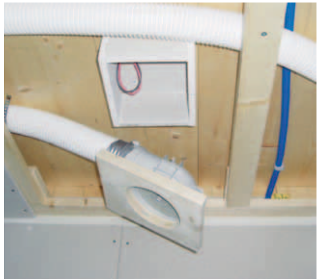
Fig. 14: Running of pipes behind suspended ceiling. System HOVAL [with the kind support of Eberle • d e n k f a b r i k • Dornbirn, Austria].
