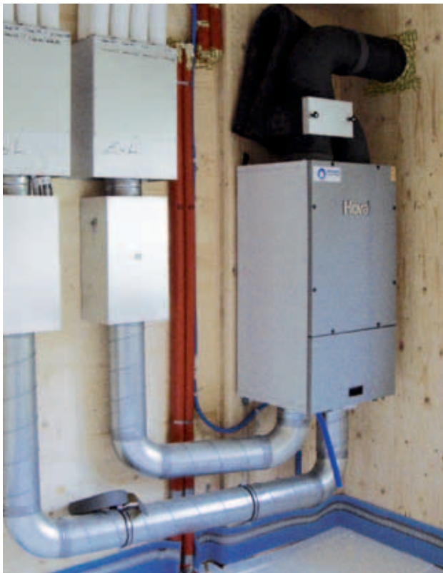
Fig. 13: Mounting of a ventilation system on a KLH wall [with the kind support of Eberle • d e n k f a b r i k • Dornbirn, Austria].
