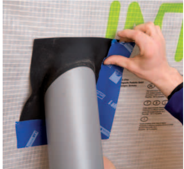
Fig. 11: If the penetrations cannot be avoided, suitable and approved systems should be used for sealing. A quick and permanently tight mounting will justify the additional costs [with the kind support of the company pro clima 2011].
