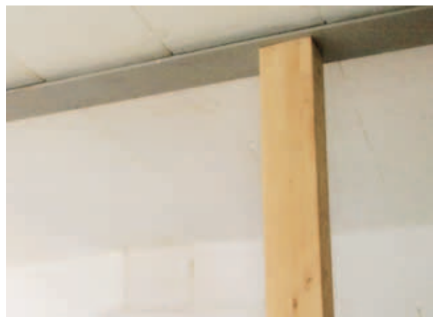
Fig. 6: A linear thermal bridge in formation. If the steel beam is not additionally integrated into the insulation, condensation is to be expected.
